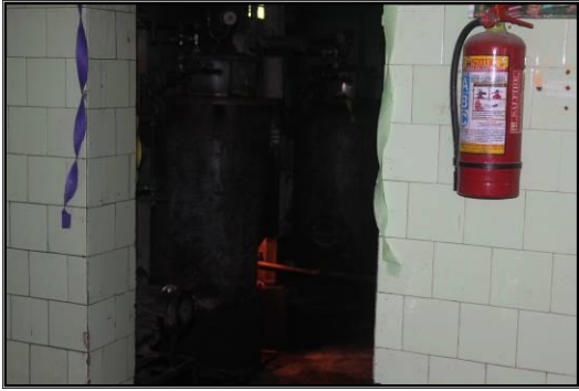
Fire extinguisher is fixed in the Central Kitchen
